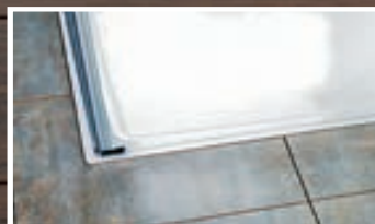
Embedded into the floor
