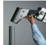
Installation of the arms with no holes
